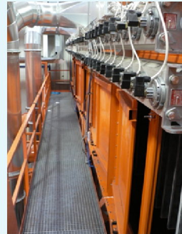
Compressed air control valves for cleaning the filter elements with compressed air
