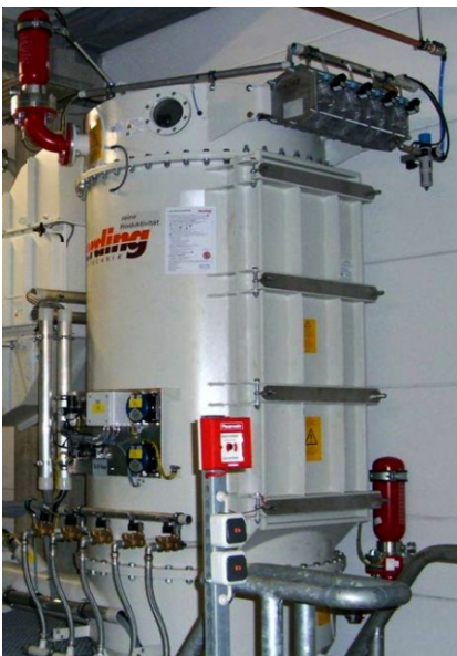
Central Vacuum Cleaner with connection to filter units and vacuum blowers
