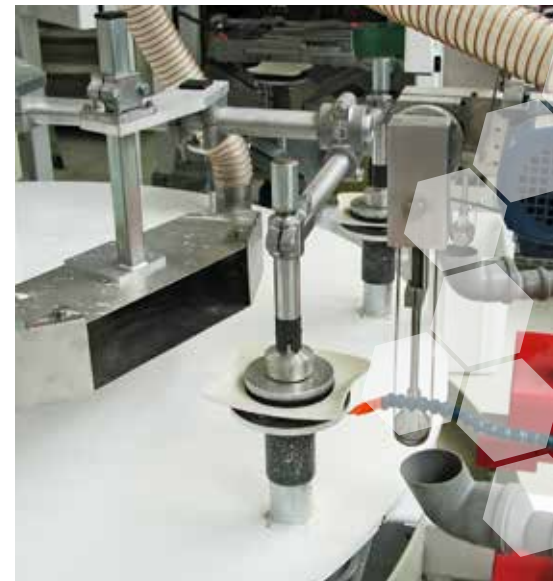
Dust capturing hoods at a fettling/rim treatment machine
